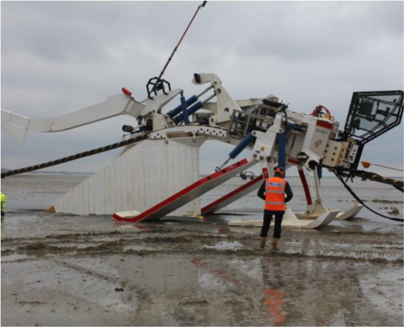
Prysmian's HD Power Cable plough (built by Soil Machine Dynamics) on Normandy Beach
